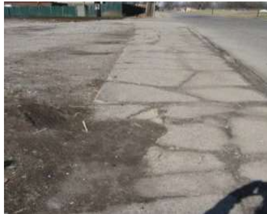
Category C-2 – Wide Cracks (>1/8")
