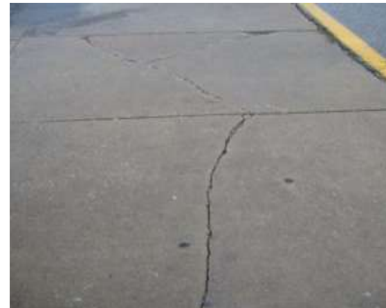
Category C-5 – Narrow Cracks (<1/8")
