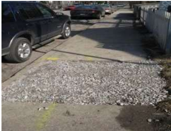
Category C-4 – Surface Defects (Concrete Spalling)
