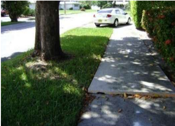
Category C-1 – Large Vertical Displacement (>1/4")
