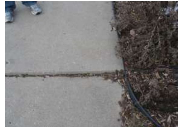
Category C-3 – Small Vertical Displacement (<1/4")
